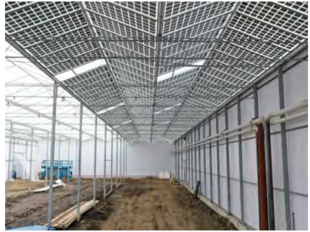
Hortisolar in Zevenbergen (NLD), 390 kWp.
