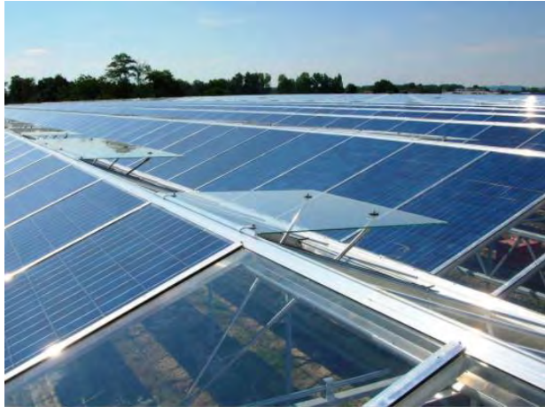
Hortisolar panels in Italy, solar roof, 2MW.
