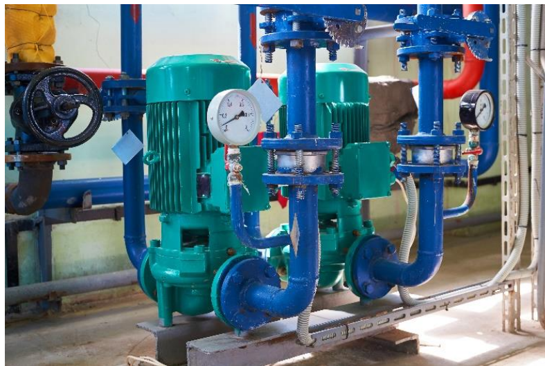
Figure 3: Pump with a three phase electric motor
