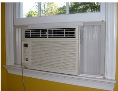
Figure 3: Example window/wall air conditioner
